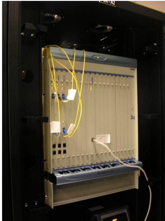
Figure 3: Optical Line Terminal (OLT) Equipment
