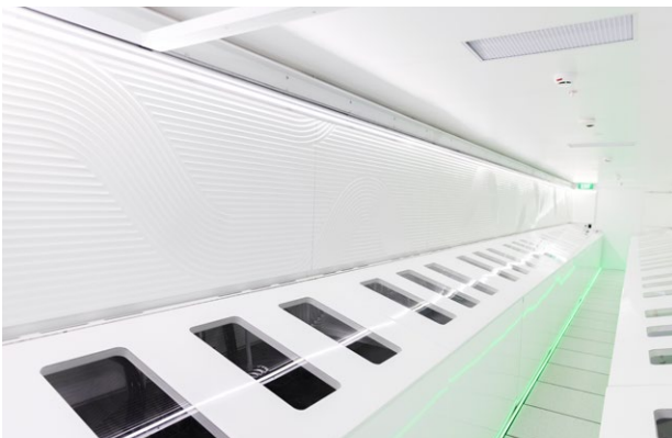
Row of immersion cooling tanks
